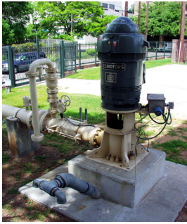
Figure 1: High-Capacity Water Well, Houston, Texas Capacity greater than 1 million gallons/day.
