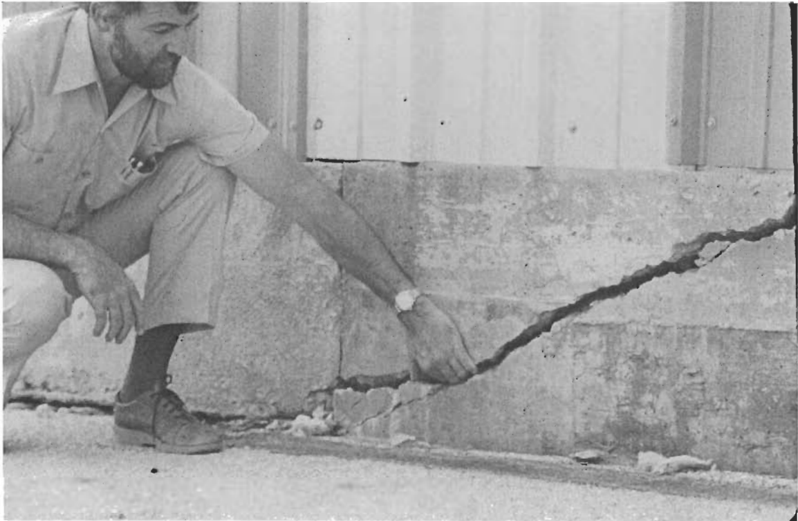
1978 – Brittmoore Fault. Crack in Foundation at Edge of Upthrown Fault Block
