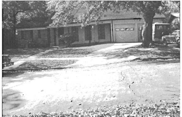
1977: House with broken foundation (photo by E. Clanton)
