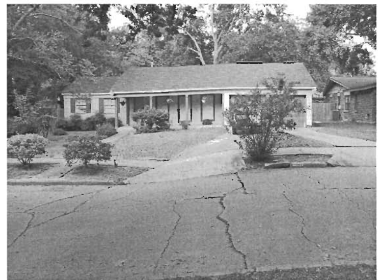
2003: House with recurring foundation problems (photo by TSI)
